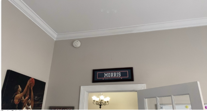
Smoke Detector Location: 34.770673, -86.778981 Date: Dec 13, 2023 12:09:19 PM CST
