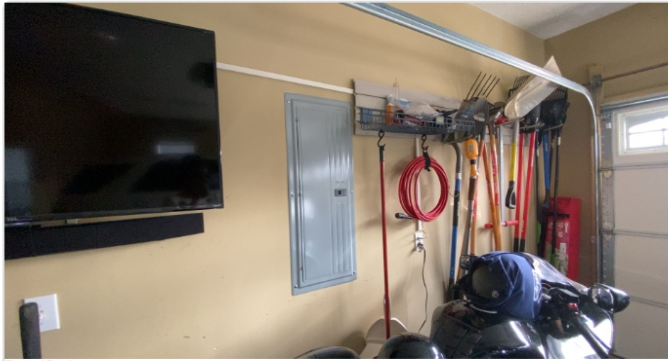
Electrical Panel Location: 34.770673, -86.778981 Date: Dec 13, 2023 12:17:11 PM CST
