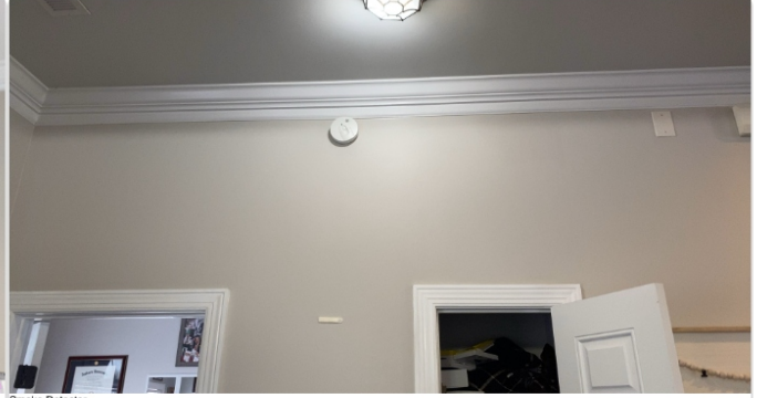
Smoke Detector Location: 34.770673, -86.778981 Date: Dec 13, 2023 12:09:42 PM CST
