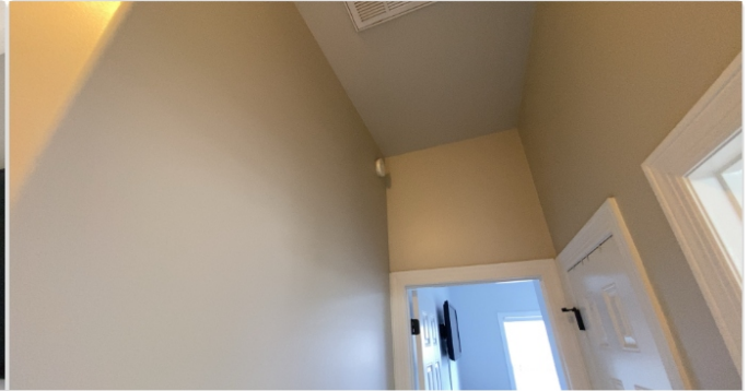
Smoke Detector Location: 34.770673, -86.778981 Date: Dec 13, 2023 12:16:26 PM CST
