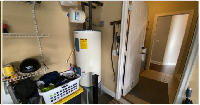
Hot Water Tank Location: 34.770673, -86.778981 Date: Dec 13, 2023 12:17:19 PM CST
