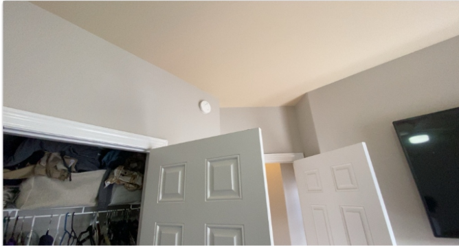
Smoke Detector Location: 34.770673, -86.778981 Date: Dec 13, 2023 12:16:12 PM CST
