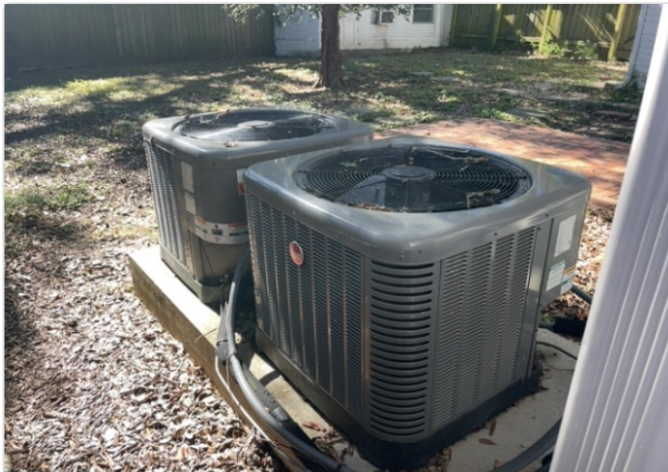
HVAC Location: 30.020510, -90.080050 Date: Dec 15, 2022 12:08:48 PM CST
