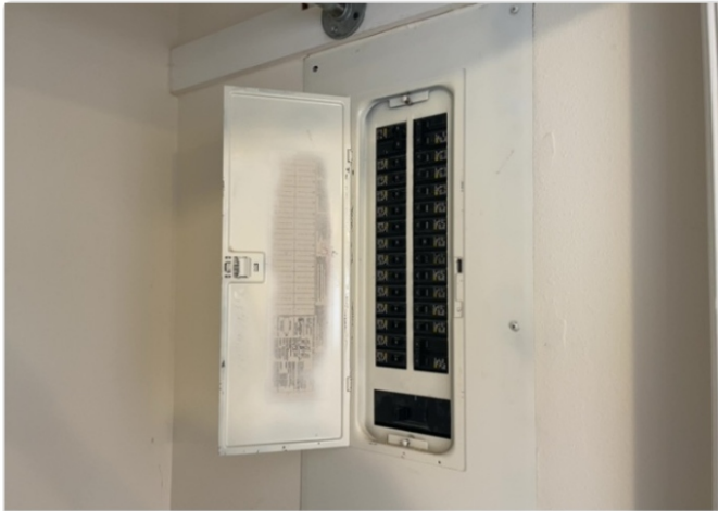
Electrical Panel Location: 30.020510, -90.080050 Date: Dec 15, 2022 12:40:25 PM CST
