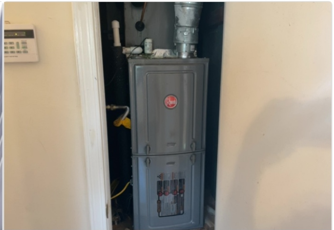
HVAC Location: 30.020510, -90.080050 Date: Dec 15, 2022 12:28:54 PM CST
