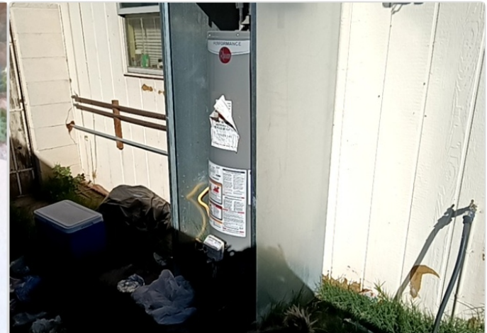
Hot Water Tank Location: 33.483398, -112.248275 Date: Feb 10, 2023 03:23:14 PM MST
