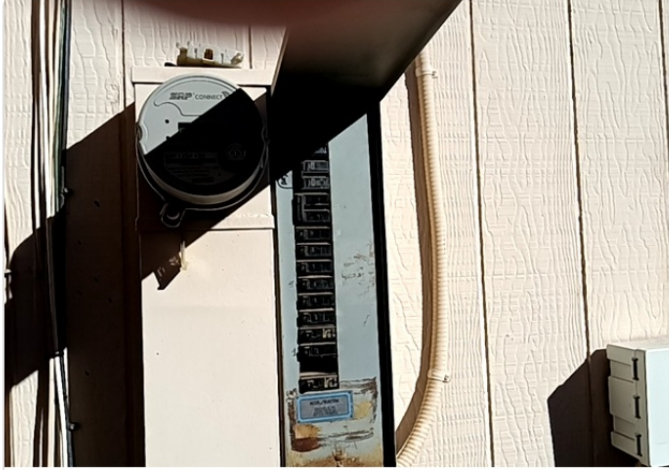
Electric Panel Location: 33.483398, -112.248275 Date: Feb 10, 2023 03:23:57 PM MST
