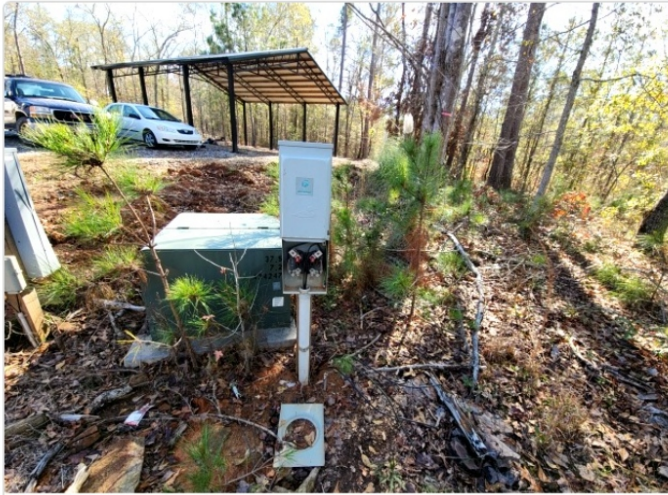
Temp power pole Location: 33.120075, -84.203684 Date: Nov 27, 2023 01:41:15 PM EST
